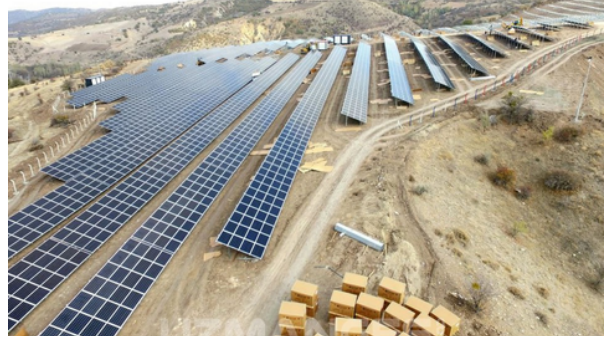
Bayburt Danişment 6 MWP
